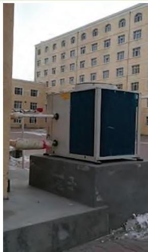
Air-to-water Heat Pump System
